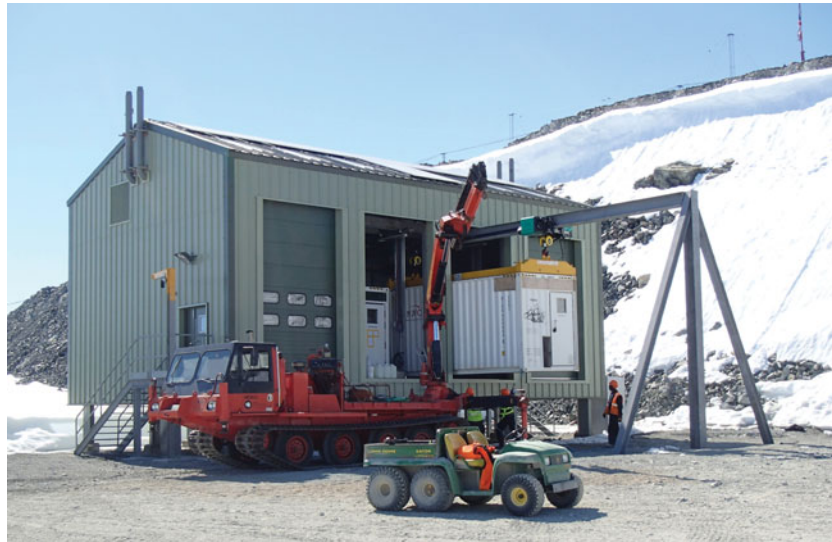
Fig. 4. The unique, purpose built A-frame gantry system for lifting and moving the units. Photo: T. Biggs
