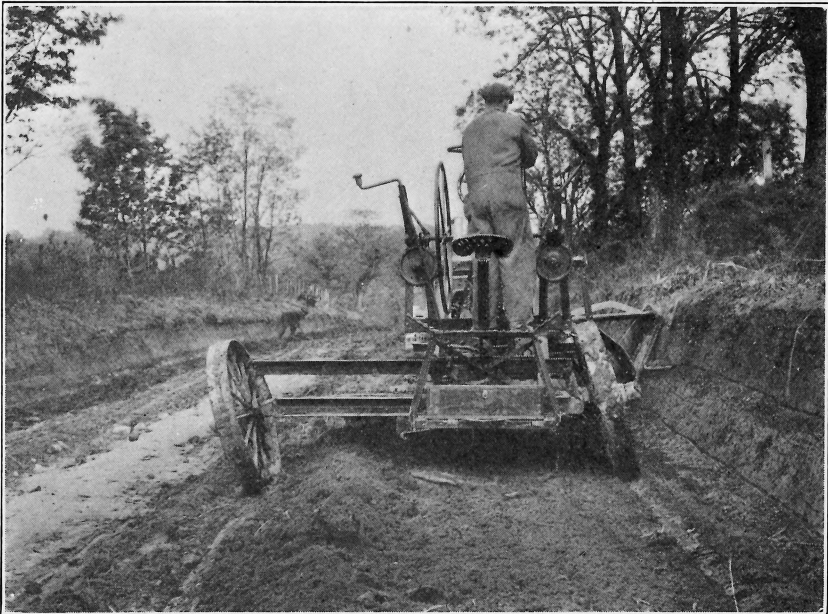
FIG. 28.— Ninth Round of Grader. This round completes the trimming of the back-slope and cuts the ditch.
