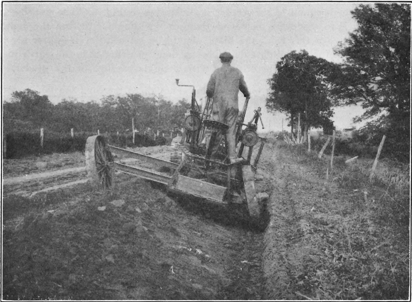
FIG. 9.— Fifth Round of Grader, Third Ditch Cut. The ditch is deepened, and the spoil delivered onto the shoulder.
