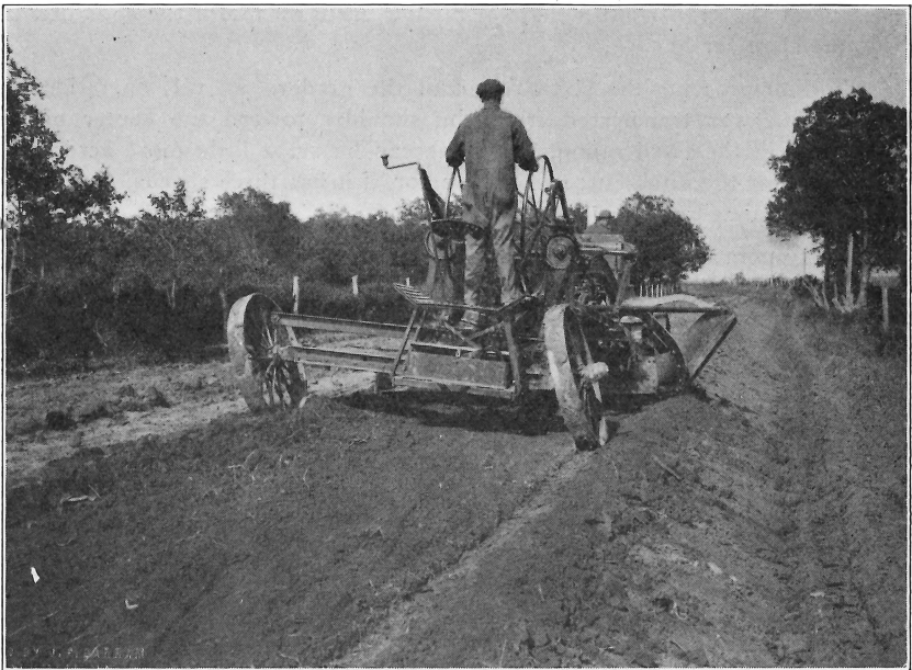
FIG. 10.— Sixth Round of Grader. The loose earth is transferred from the shoulder toward the center of the road.
