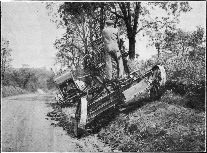
FIG. 20.— First Round With the Grader. The cutting of the banks is started at the top of the slope.
