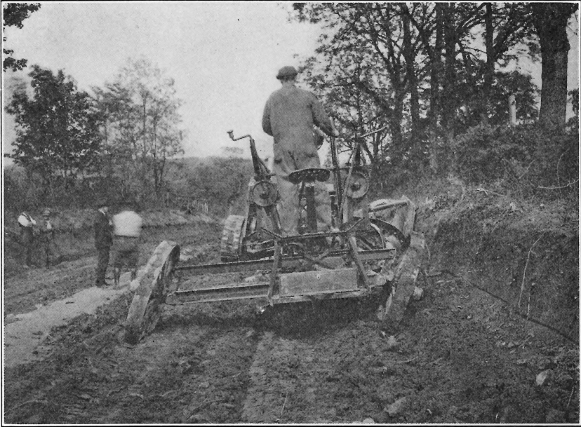
FIG. 27.— Eighth Round of Grader. The trimming of the back slope is continued in this round.
