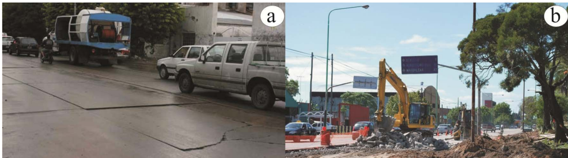
Figure 1: (a) Pavement affected by longitudinal and transverse cracks, slab sinking and joint faulting. (b) Removal of concrete slabs (sampling area).
