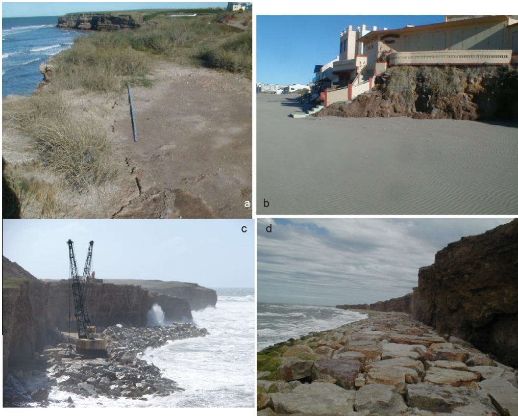
Figure 4 - Cliffs from Mar del Plata (38° S, see figure 1 for location). a) Fracture cracks on the top of the cliffs. b) Sea-side constructions are usually located attached to the cliffs composed of indurated siltstones. c) Rock revetments under construction. d) Armored structures are today protecting some cliffs.
