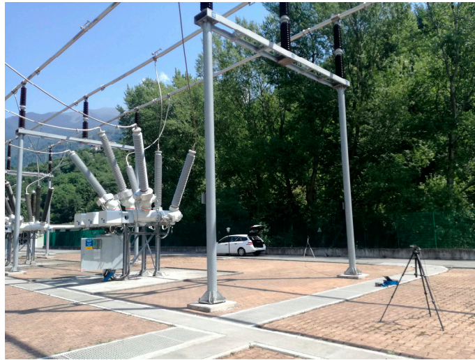
Figure 4. Example of TSG installation in a high-voltage substation.
