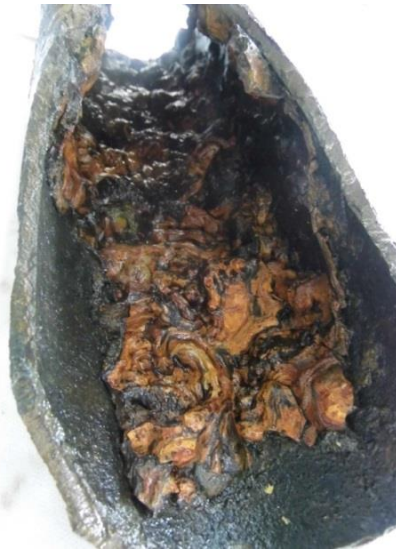
Figure 3-6. Inner walls of cast iron pipeline of sampling point 2
