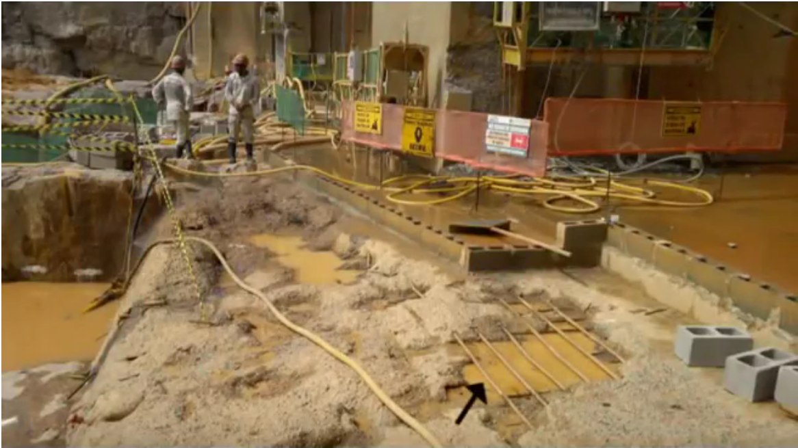
Fig. 5.10 A photograph showing the dam wall after the dam had been drained, copied from [33]. Exposed re-enforcing bar can be seen in the foreground.
