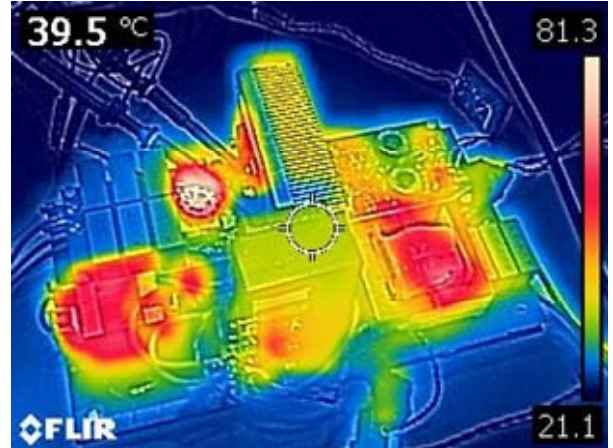
Fig. 11. Thermal photograph of circuit in Fig. 8. The temperature of H1 is registering as lower than its actual temperature due to the low emissivity of its surface. The actual temperature of H1 was measured at approximately 52^\circ\text{C} with a thermocouple.
