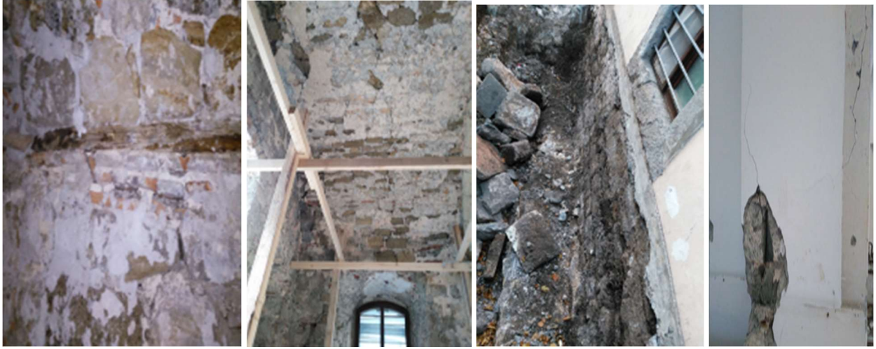
Fig. 4. Views from damages in the mosque
