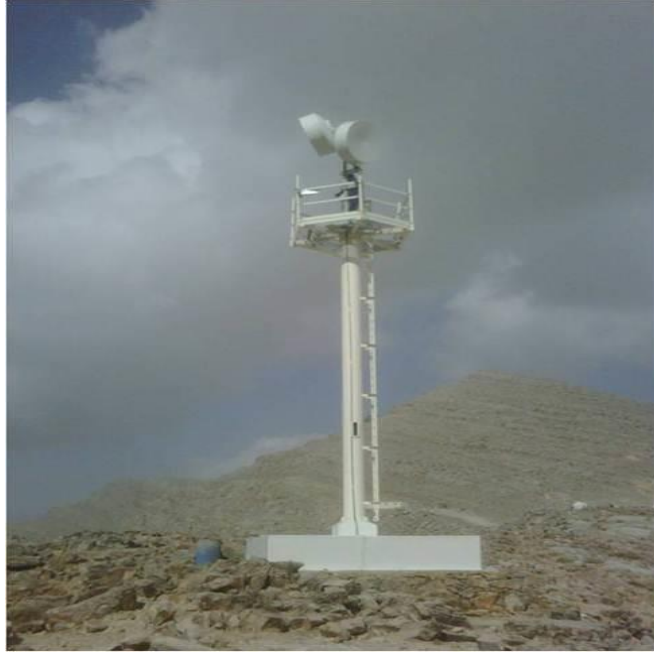
Figure 3.5: Fixed Antennas over the Top of the Tower
