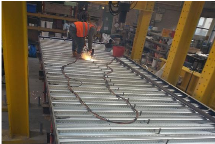
Fig. 3 Welding of shear studs to the steel beam flange through the decking
