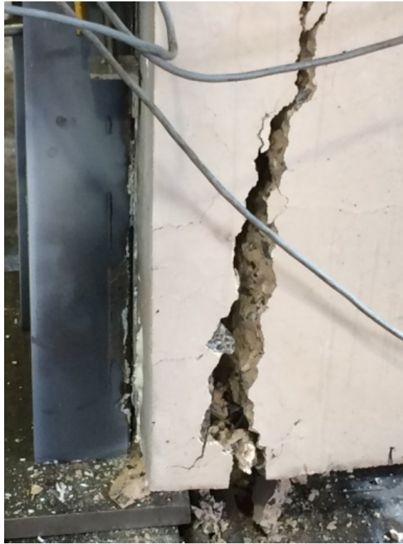
Figure 14. Failure mode of Blind Bolt 2 connector specimens post fire
