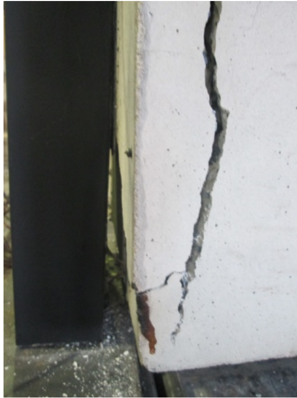
Figure 10. Failure mode of Blind Bolt 1 connector specimens post fire
