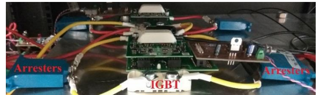
(a) The IGBTs and the arresters in the main breaker path
