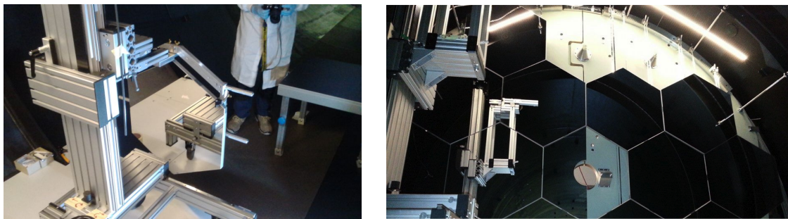
Figure 16. Left: installation tool with a hexagonal mirror ready to be mounted. Right: mirror mosaic close to completion (only two hexagonal mirrors on the top right are missing; the installing tool is visible on the left).
