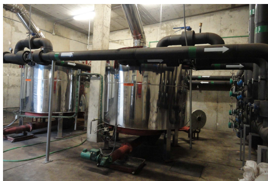
Figure 2. Thermal power plant installed in the building of Mérida (Badajoz)
