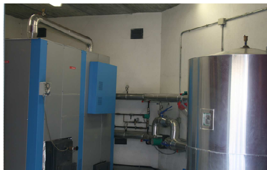
Figure 1. Thermal power plant installed in the Hospital of Zafra (Spain)
