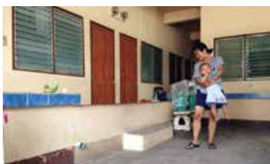
Fig. 3 A 70 cm cement wall was made at the entrance of apartment to prevent flooding (No.9).
