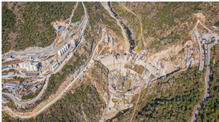
Figure 2: Excavated area due to the dam construction in Foz de Tua. (Adapted from Google Earth, 2017)
