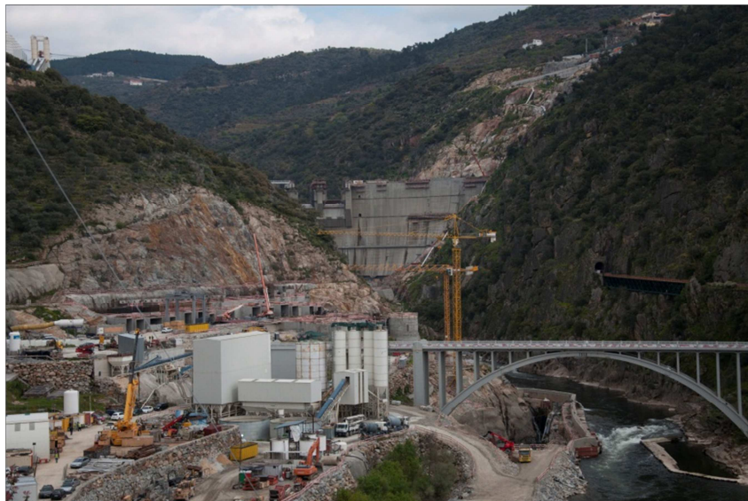
Figure 6: Perspectives of the Foz de Tua dam during construction phase. Photo by Paulo Cortez
