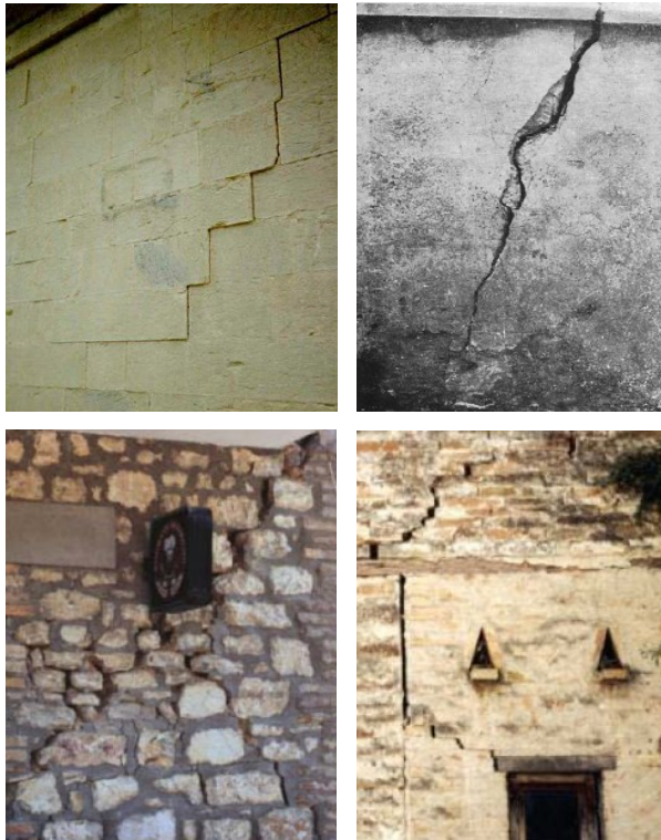
Fig. 1.2 - Some typical failure modes of the first type: detachments.
