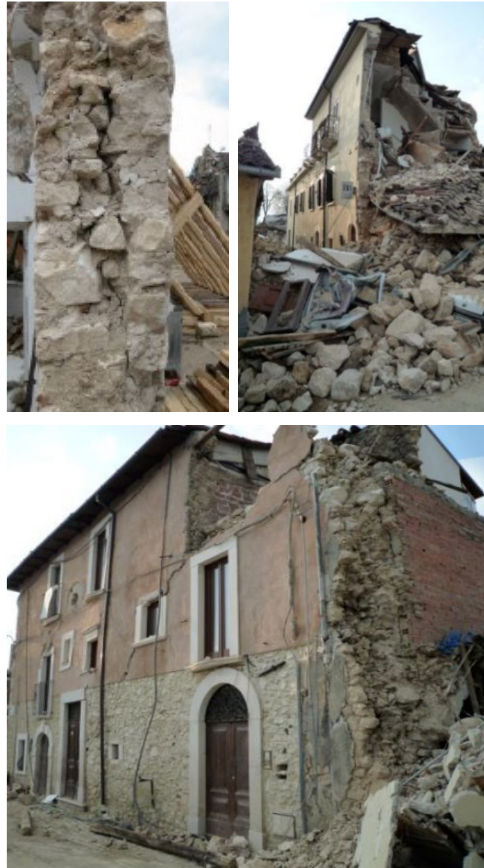
Fig. 1.7 - Examples of poor quality masonry (Onna).
