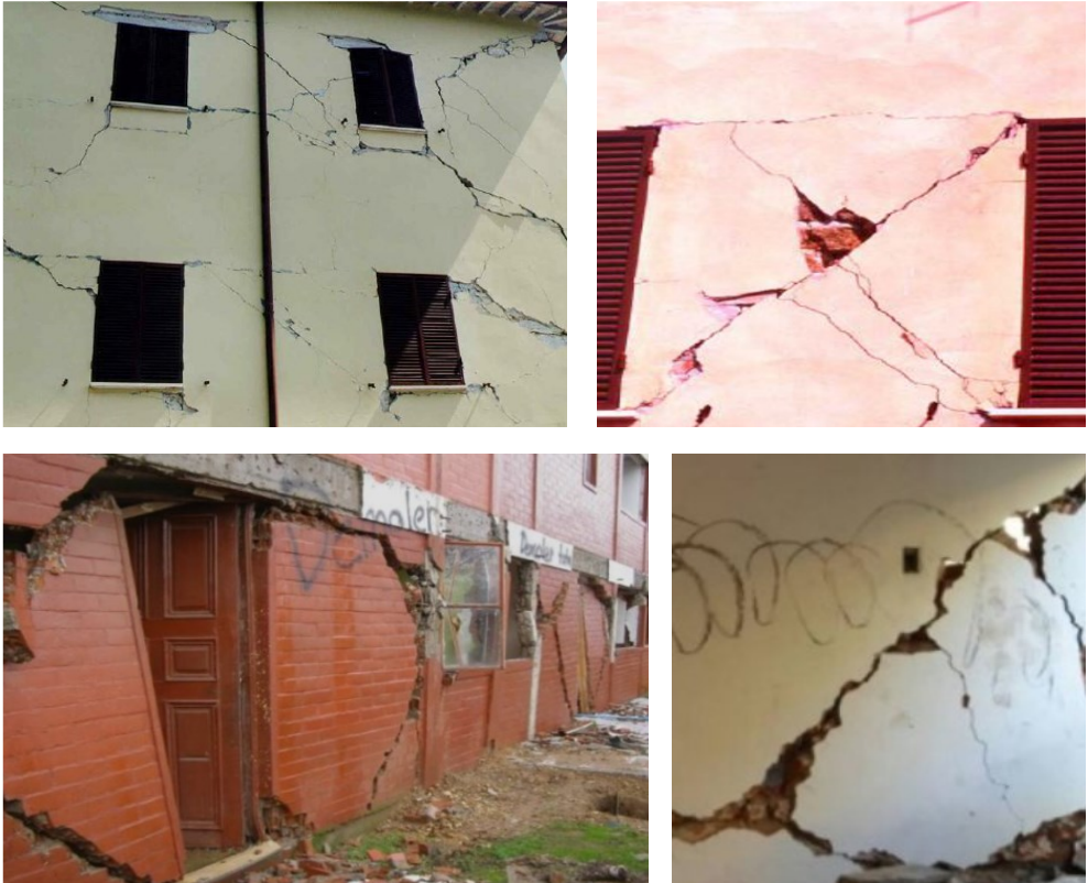
Fig. 1.4 - Some typical failure modes of the second type: detachments and sliding. These fractures occur when the structure is close to collapse (e.g. under seismic action).
