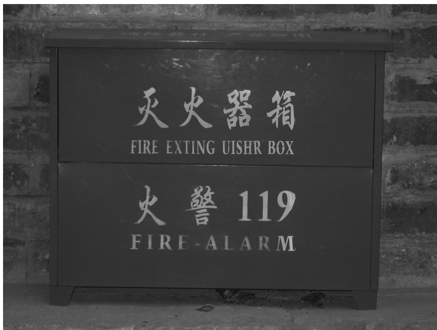
Figure 1.1 'Fire Exting Uishr Box'
