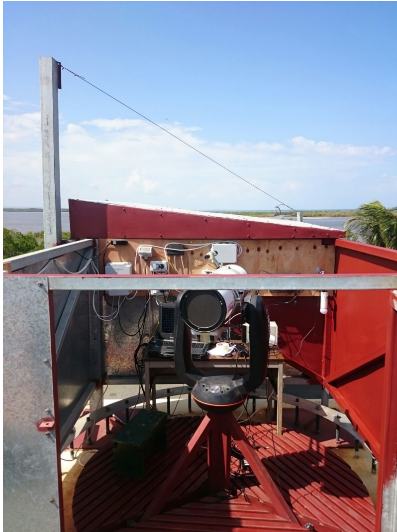
FIGURE 2.4: EQUO-OG installed at Broglia Space Center.
