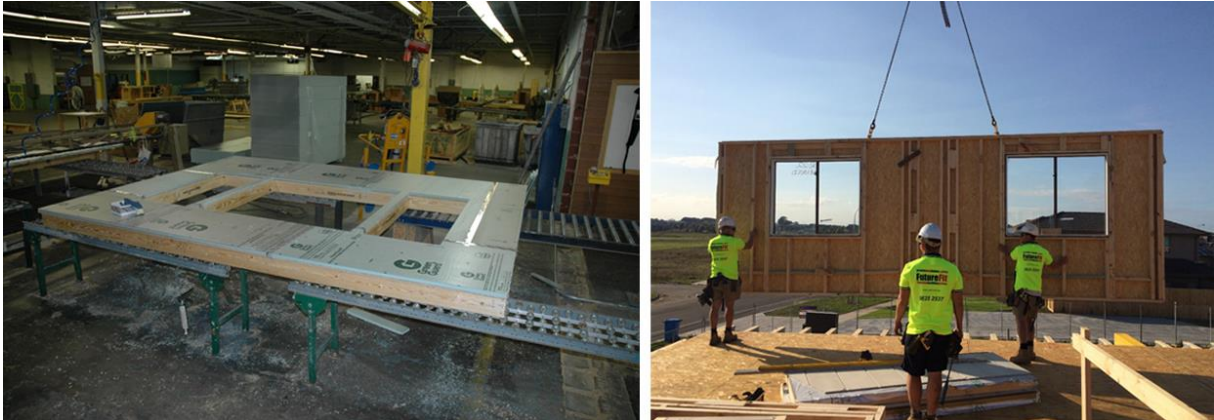
Figure 2-5: (Left): Panel preparation in Factory with openings already cut and prepared, (Right): Erection in site using cranes and trained workers. Source: Left - https://www.oremonte.org/enchanting-panelized-homes-texas/ , Righth: prefabaus.org.au
