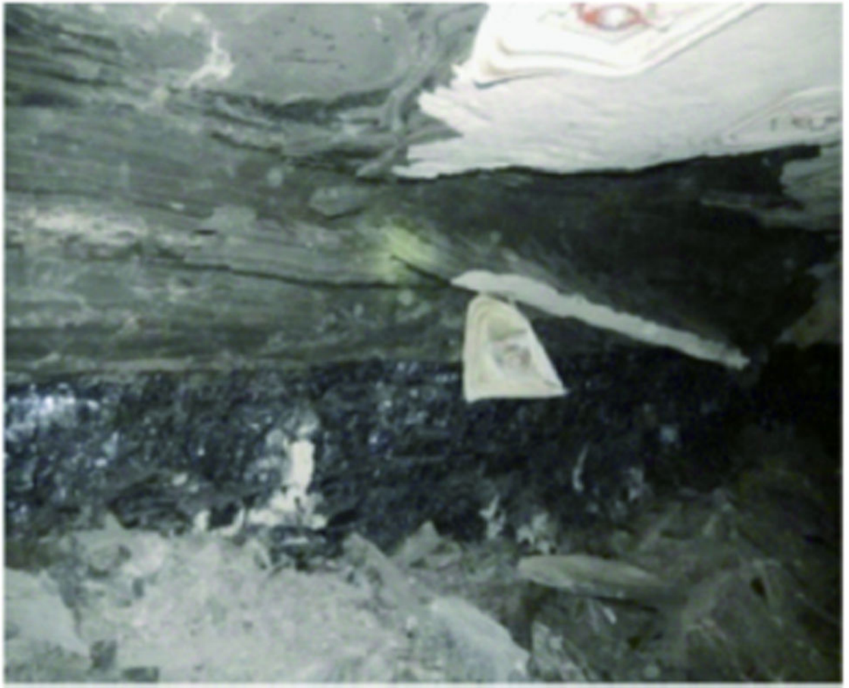
Fig. 19. Rib sloughage at the panel side in the bleeder entry of Panel II in the lower seam.
