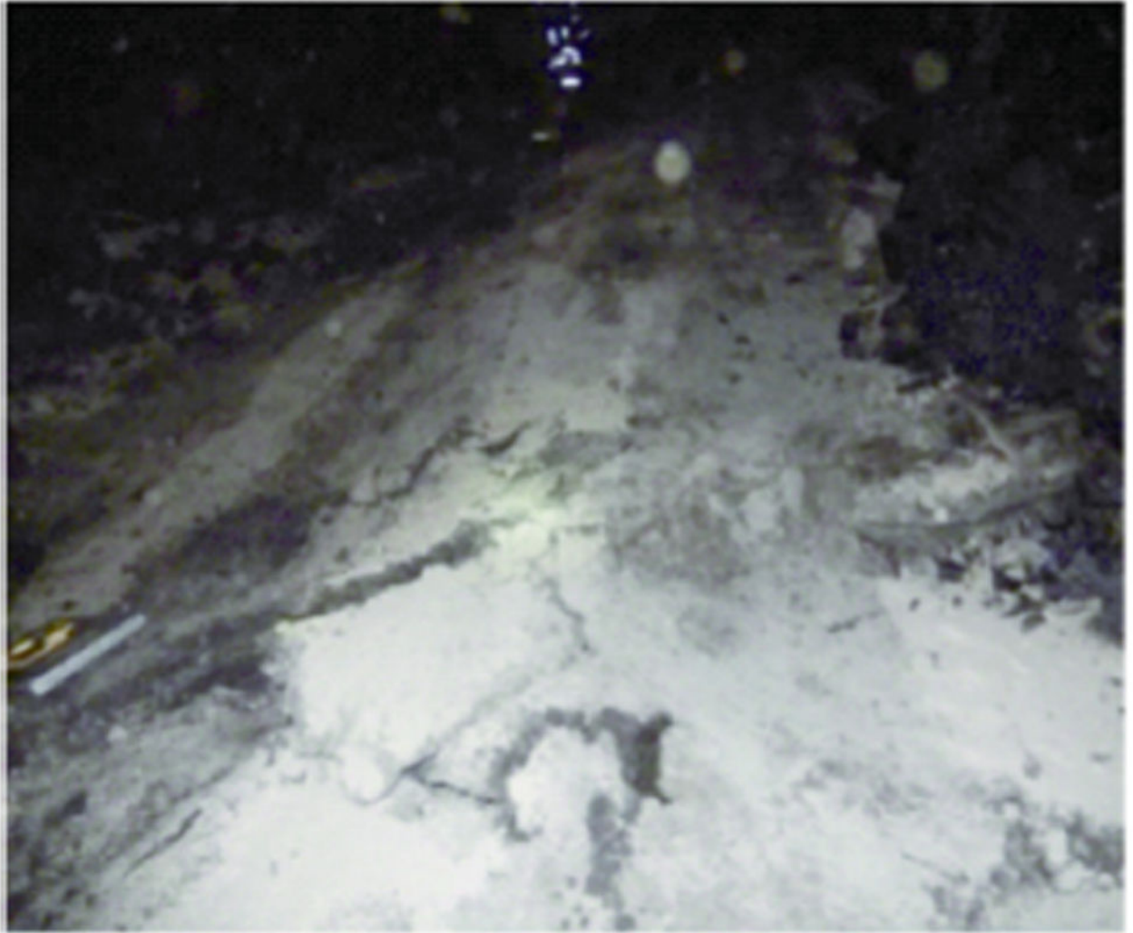
Fig. 21. Floor heave in the bleeder entry of Panel II in the lower seam.
