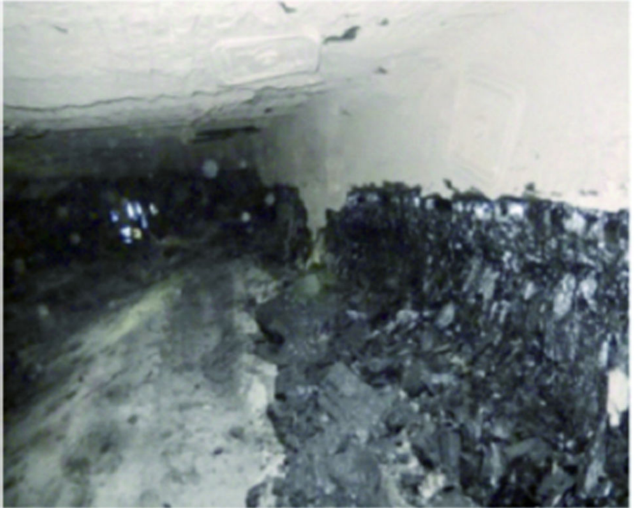
Fig. 20. Rib sloughage at the barrier side in the bleeder entry of Panel II in the lower seam.
