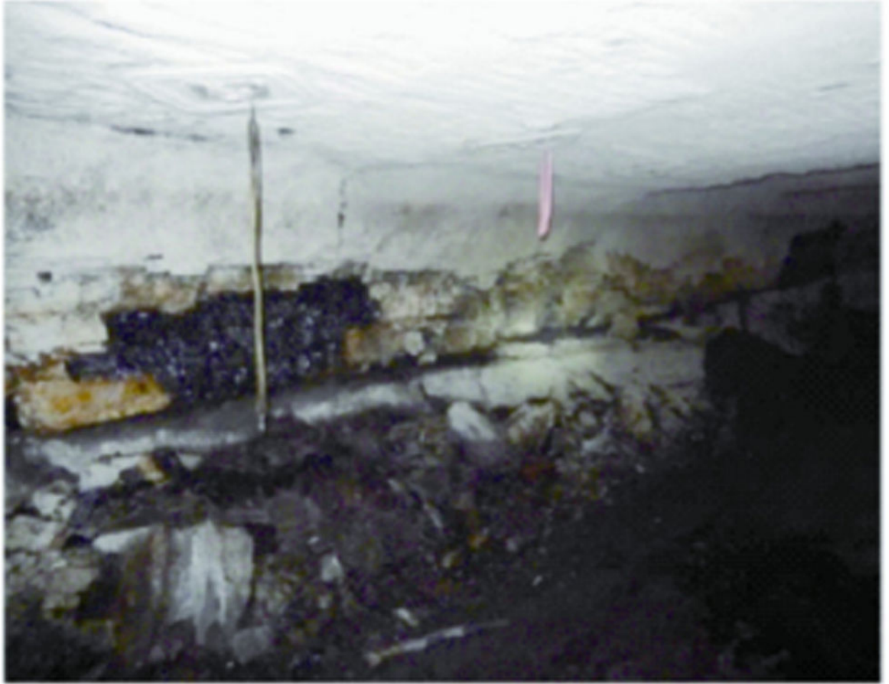
Fig. 15. Rib sloughage outby the pillaring line during retreating in the upper seam.
