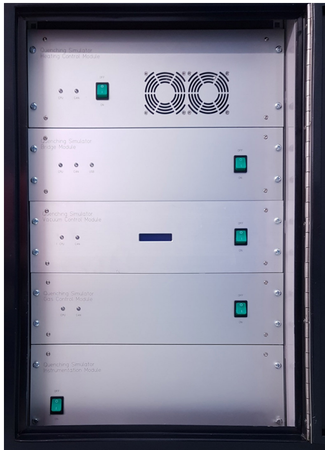
Figure 3.77 - The individual module enclosures installed in the main instrument enclosure.
