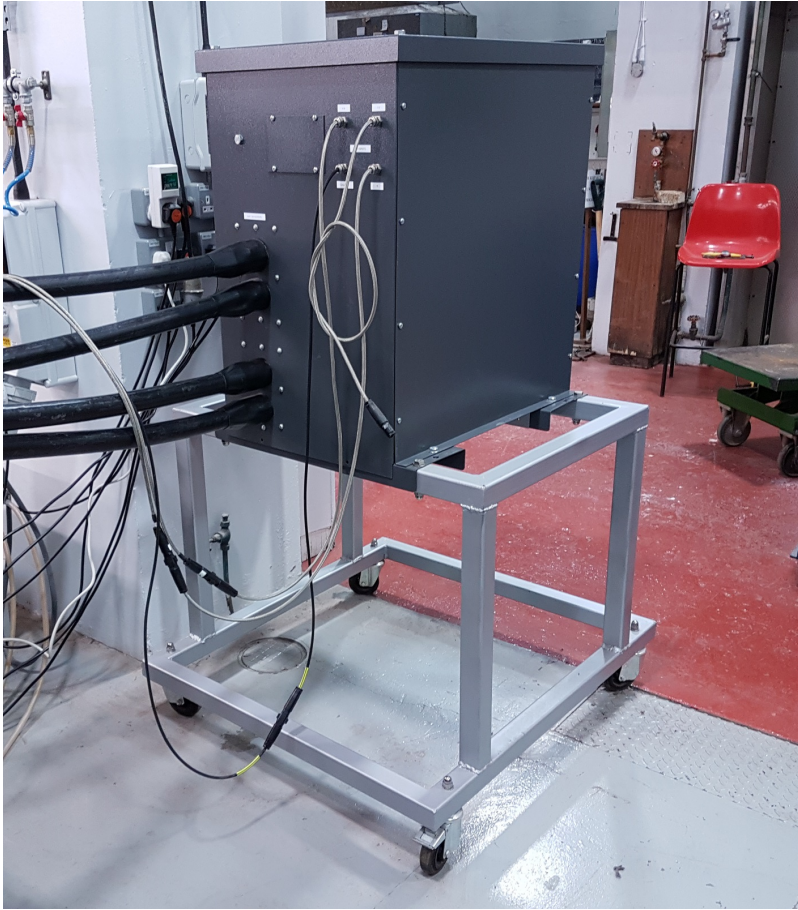
Figure 3.78 - The power transformer and support frame.
