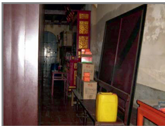
Figure 8. The flammable materials and substances are not well-kept
