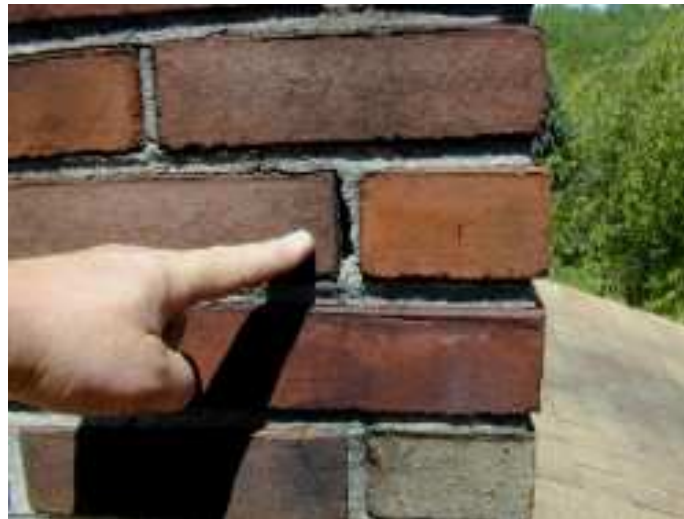
Figure 1. Problem of worn mortar joints
