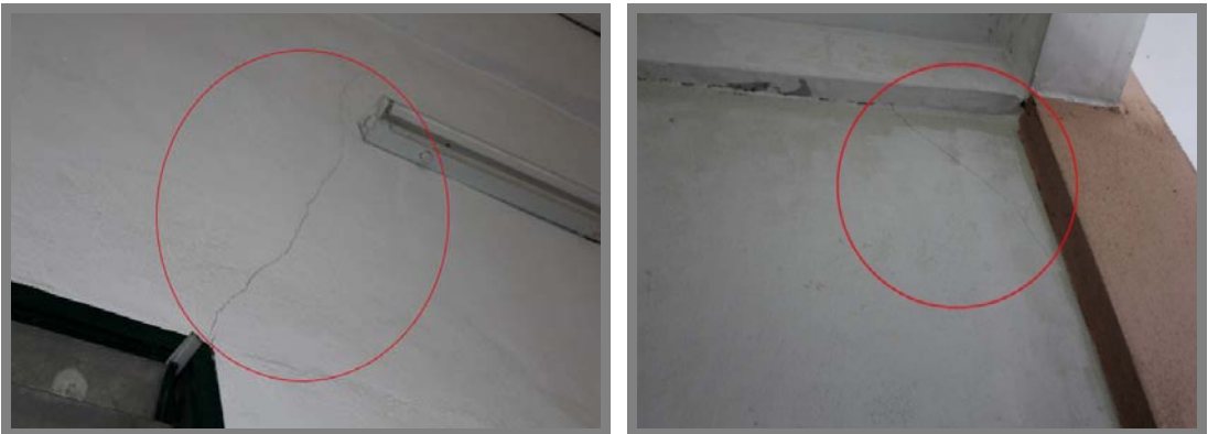
Figure 5: Diagonal crack on wall and at the corner of door
