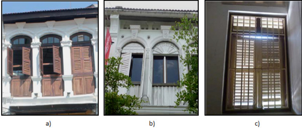
Figure 6: Actual condition of façade at Rainbow Lodge, Red Inn Penang and Red-Inn Heritage buildings a) Missing balustrade-Rainbow Lodge b) secondary window-Red Inn Penang c) cast iron grill-Red Inn Heritage
