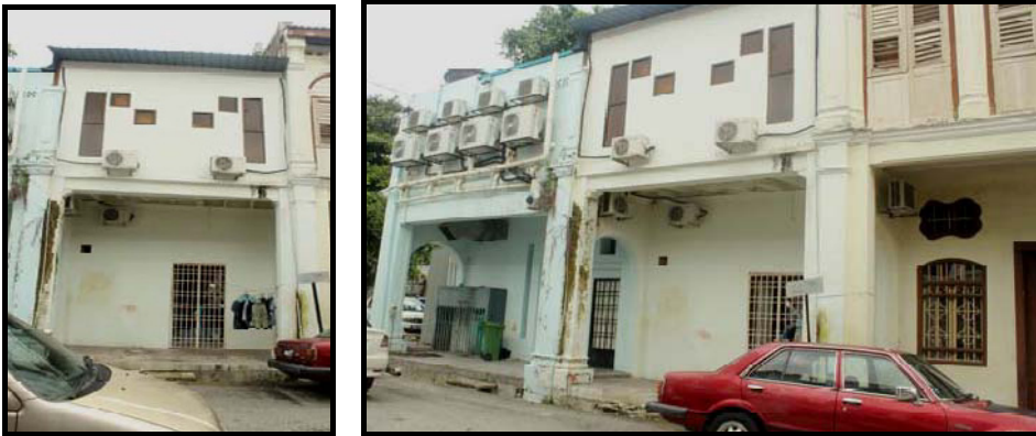
Figure 14: The appearance of the rear façade and the opening which is totally different from the front façade and adjacent buildings
