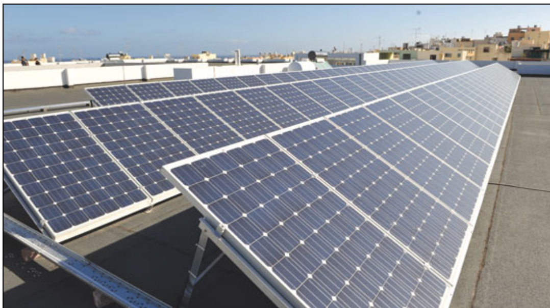
Figure 3.1: Photovoltaic panels installed at Pembroke Primary School. 144
