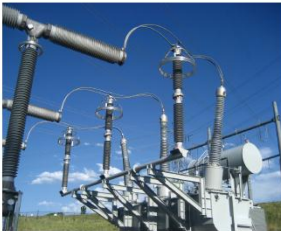
Figure 19: Metal Oxide Varistors (MOVs) mounted on transformers for lightning protection also moderate the effects of E1 171
