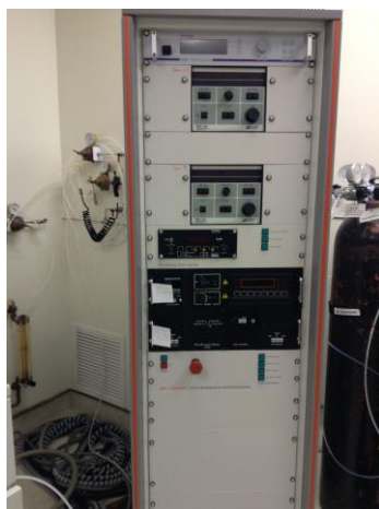
Magnetron Control Center
