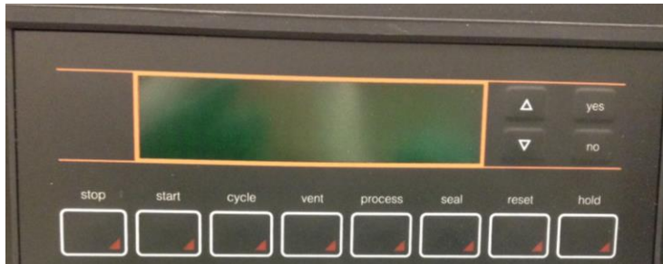
Vacuum System Control Panel
