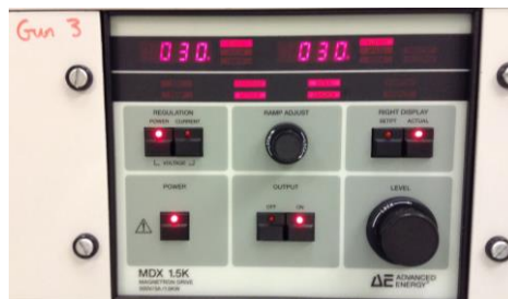
DC Power Supply
