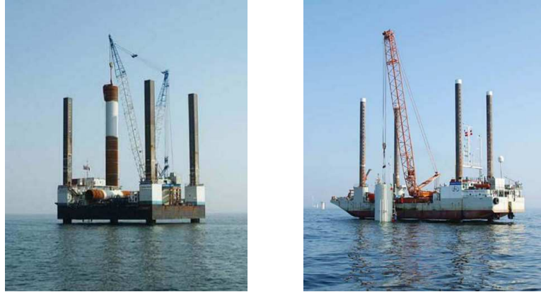
Figure 14: Jack up platform from Ballast Nedam that was used to drive in the monopoles for the Horns Rev wind farm. 91
