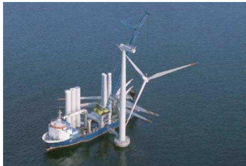
Figure 17: Crane barge EIDE V used for the installation and construction of the foundations and turbines for the Nysted wind farm. 109
