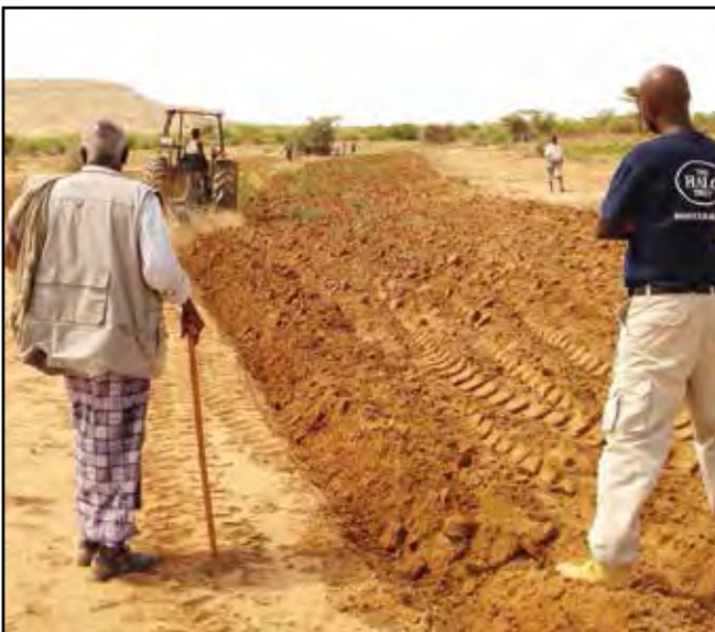
An area is cultivated following clearance by HALO. Photo courtesy of The HALO Trust.
