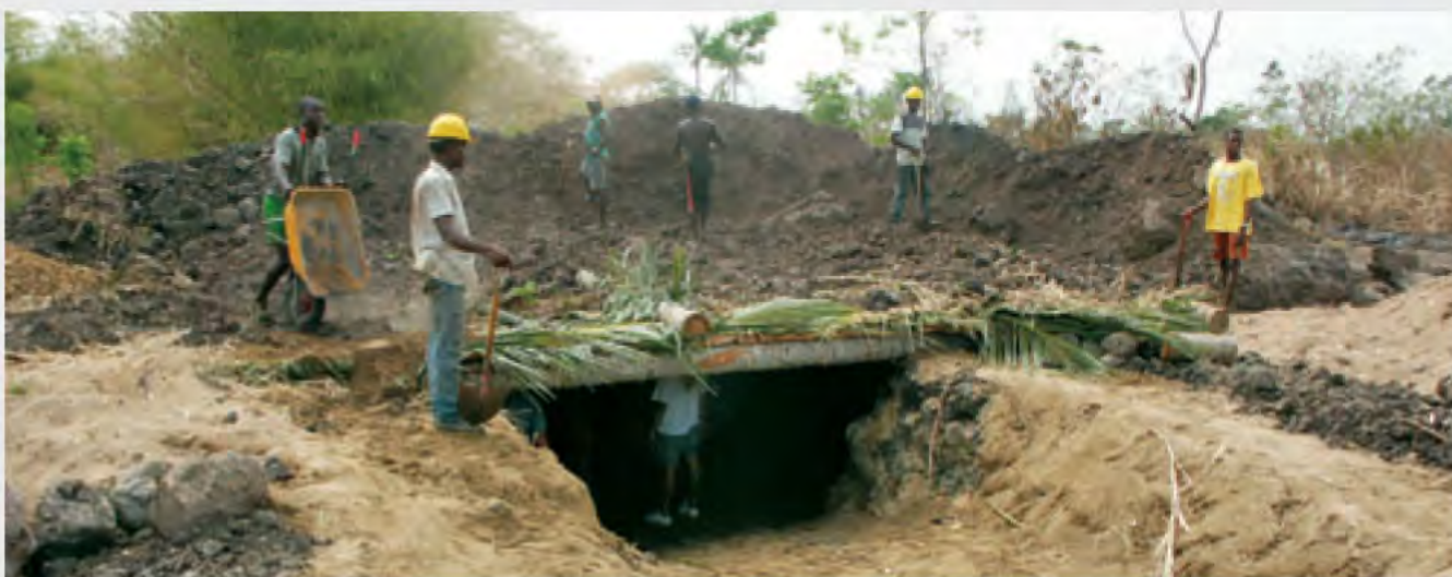
Workers repair a firing pit at a government demolition range so that arms and munitions excess to the defense needs of São Tomé and Príncipe may be destroyed.
