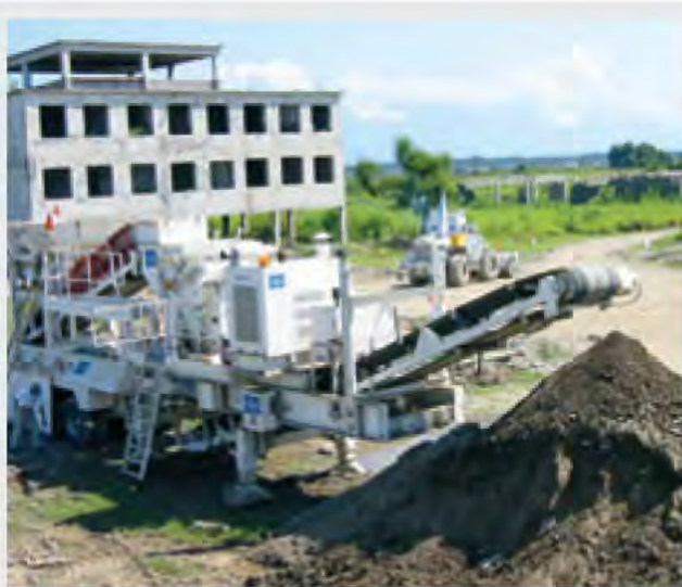
A mobile crushing machine crushes and processes earth contaminated with landmines and then deposits clean soil at the end of the conveyer belt. In the background, an armored tractor travels to a nearby location to scoop more topsoil and have it similarly processed. The HALO Trust operates both pieces of equipment in Georgia.
