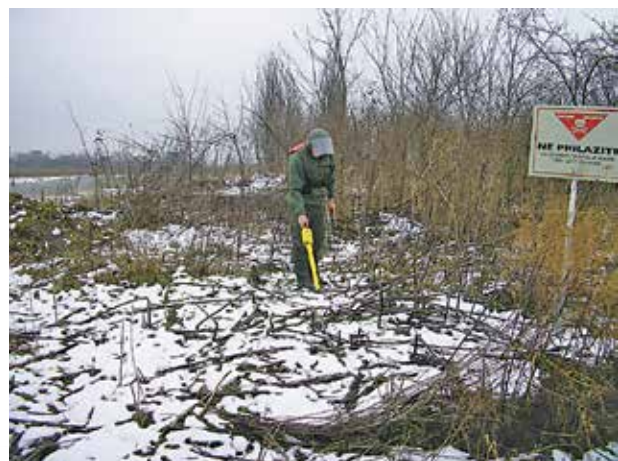
The Croatian Mine Action Center (CROMAC) employed the Schonstedt GA-72Cd locators on clearance projects along the power line in eastern Croatia near the Osijek city in very difficult terrain. Photo courtesy of CROMAC.
