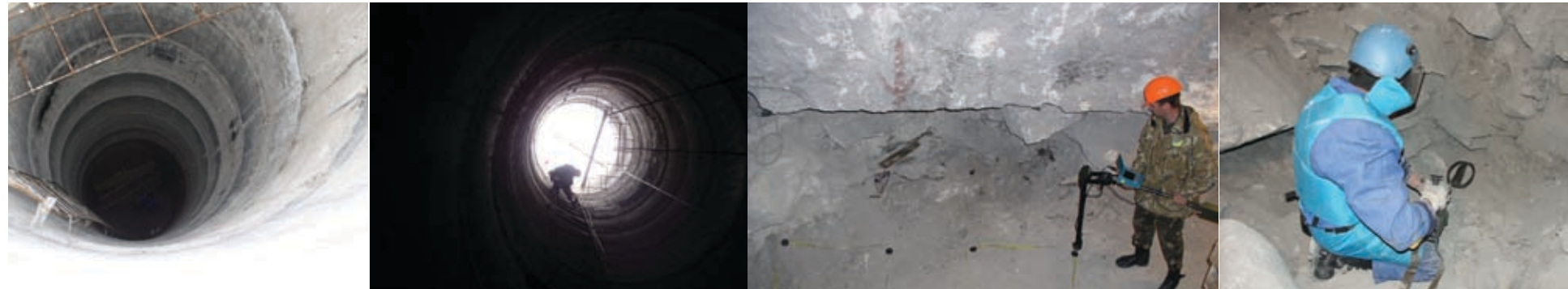
During Stage One, shaft-sinking and tunneling provide underground access. After this step has been completed, stepladders are replaced by special loading equipment.
