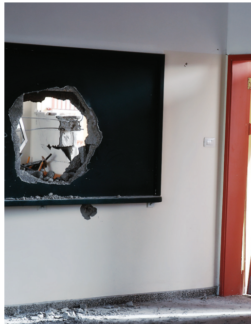
Damage to a classroom in a Balgis al Yemen school, one of the many buildings investigated by the Technical Assessment team.
