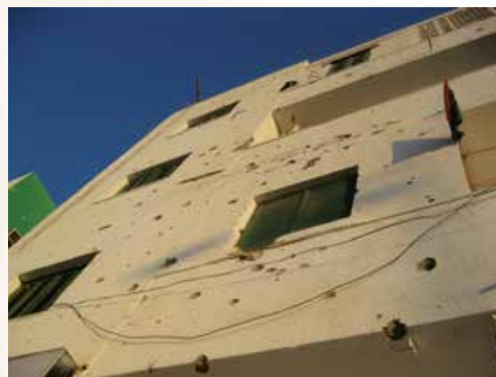
An example of low amounts of battle damage. No items of UXO were found around this building.
