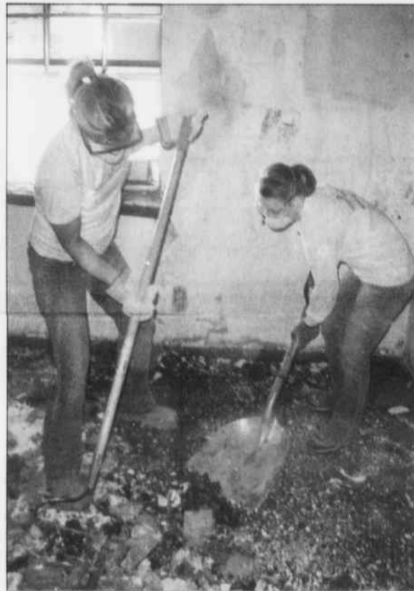
ABOVE: Chelsea Skotchdopole and Carrie Miller help restore a house. BELOW: Melinda Harvey and Miller shovel debris.
