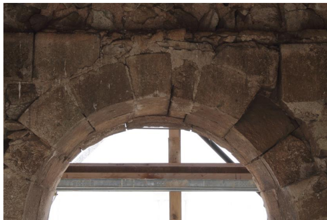
Figure 2 Internal disconnection of the keystone of an opening in the belfry.
