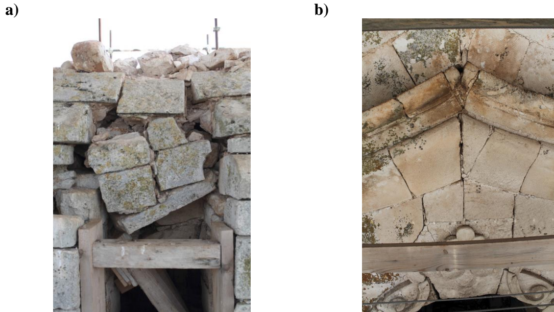
Figure 3 Disconnection a) at the basement level of the spire collapsed because of lightning; b) at the level of the keystone of an opening of the belfry.
