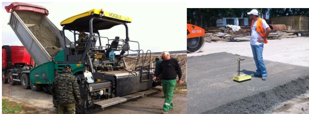
Figure 1 Left: Truck unloading onto paver and RCC laying Figure 2 Right: Fresh concrete density measured with nuclear gauge
