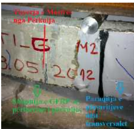
Fig.5.5.Cracking under flexure force and shear force; Set C/beam 1
