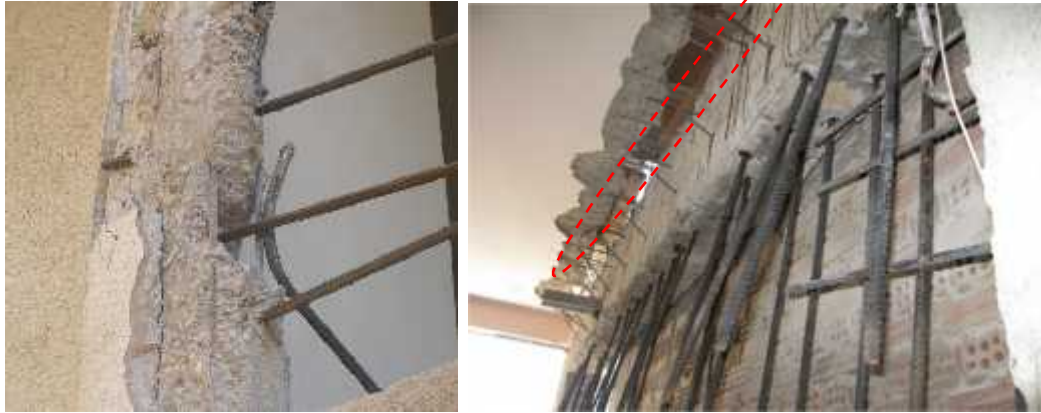
Figure 6 a-b. Misapplications of Anchors (photo a: A. Sarı ın, photo b: M.A. Özen)
