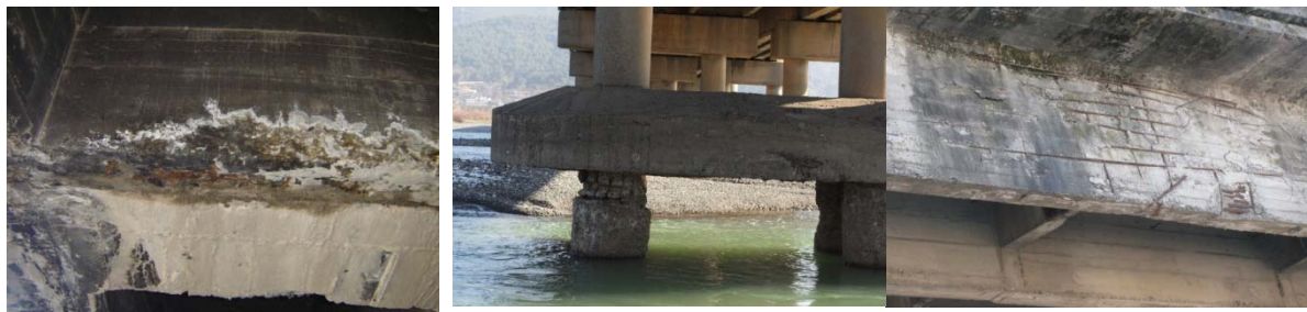
(a)Water leakage and chemical attack (b)Poor workmanship and bad construction practice (b) Heavy Scouring and chemical attack on piles' concrete
