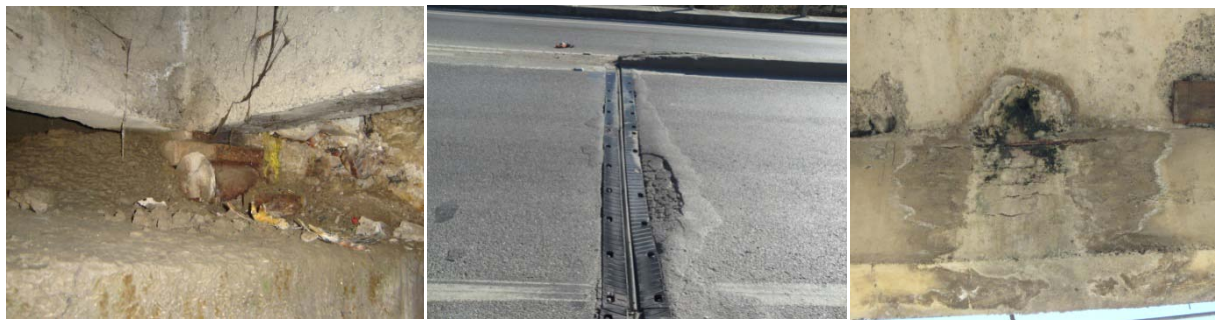
(a)Corroded & Frozen Bearing b)Defected Expansion Joint (c) Failed drainage system
