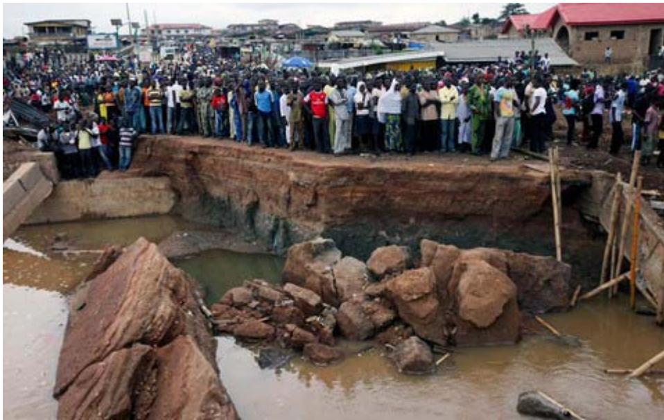
Fig. 2: Flood disaster and bridge wreckage, Ibadan (Source: http://safeafricagroup.com/2011/09/01/flood-disaster-in-nigeria/ ).
