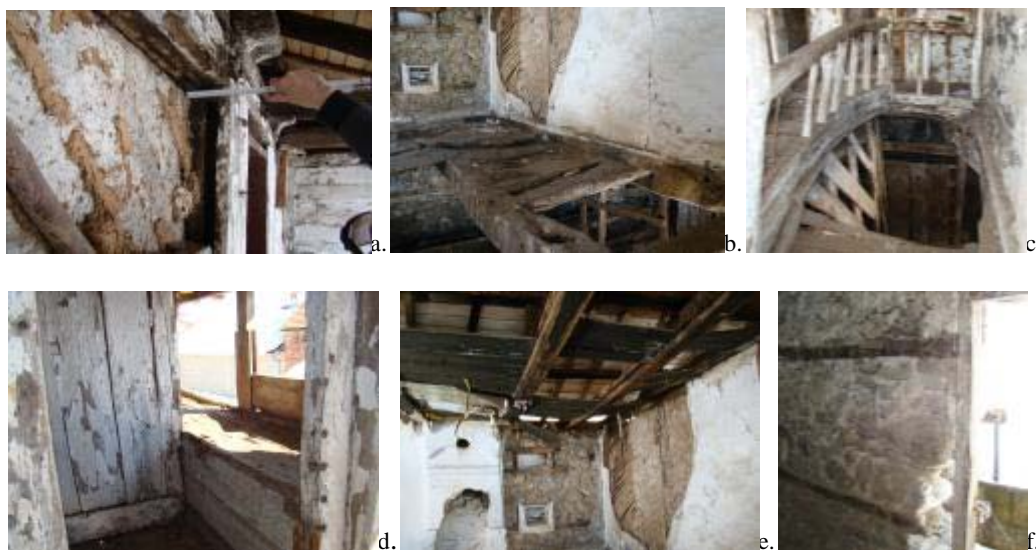
Fig. 3: a. Damaged internal wall constructed by clay reinforced with timber willows; b, c. & e. deterioration of a timber elements at ceiling/flooring and staircase structure; d. poor maintenance of planking envelope; f. misapplied of structural conservation.
