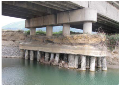
(a) Pile erosion
