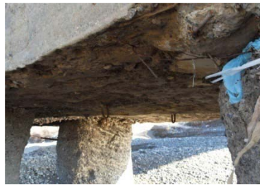
(b) Pile cap bad workmanship
