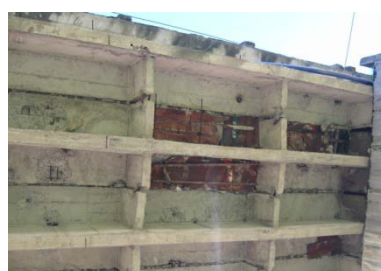
(a) Improper framework
