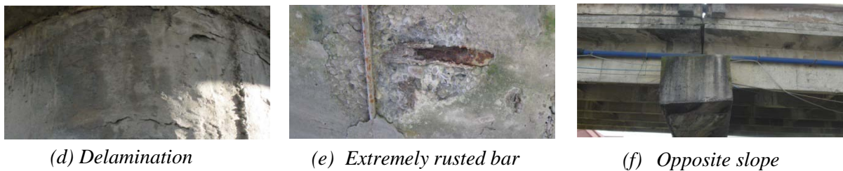
Figure 4 Pier and beam cap defects
