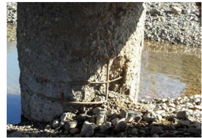
(c) Pile concrete deterioration
