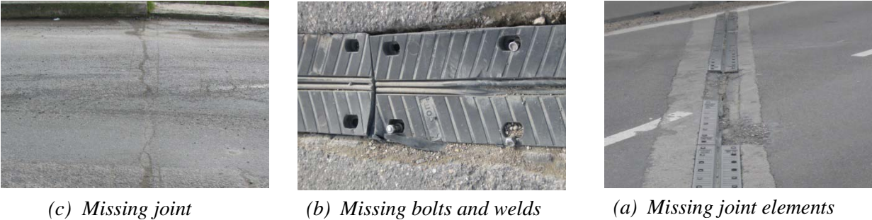
Figure 6 Expansion joint defects
