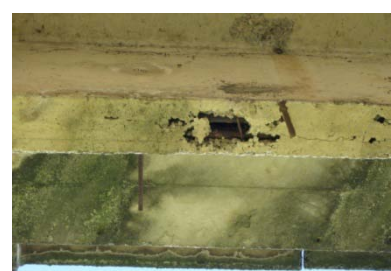
(c) Dense bars, concrete gap
