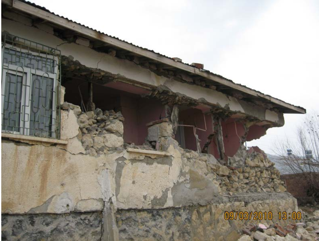
Figure 6 Damade due to the insufficient connection of the walls to each other
