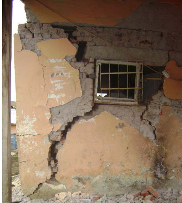
Figure 8 Wall opening close to the building corner
