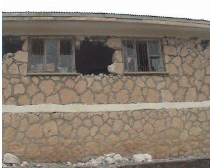
Figure 7. Damage due to insufficient distance between two openings
