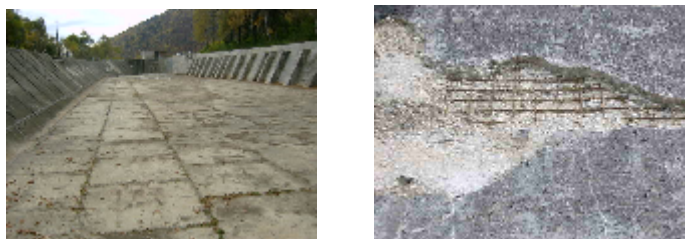
Fig.2. The view of the accumulations basin and degradation of concrete in concrete campades
