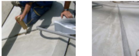
Fig.7: a/ placing the MAPEFOAM in joints; b/the view of joints after finishing
