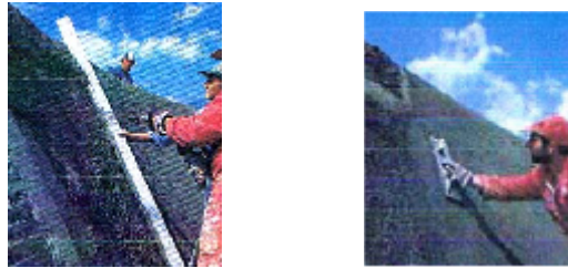
Fig.6. The cast in place and final smoothing the layer on the slope surface
