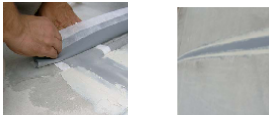
Fig.8: a/placing the PVC materials to protect the joints; b/the view of protected joints
