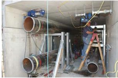
Figure 4: Inner View of the Utility Tunnel of United States Capitol Visitor Center
