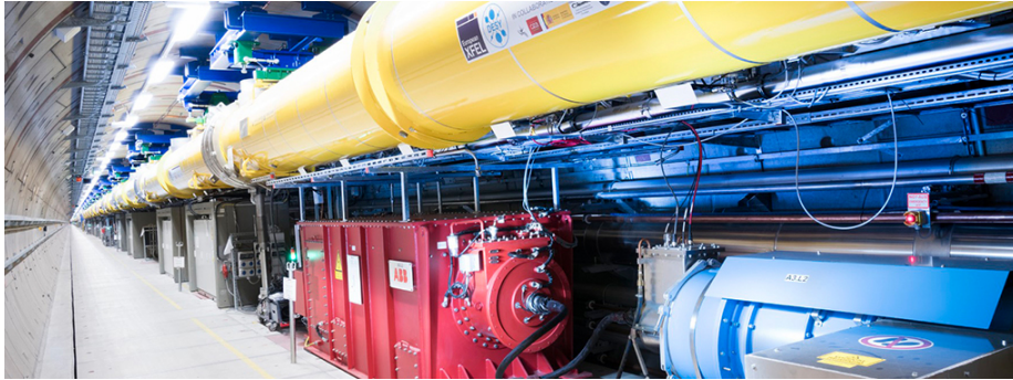
Figure 2.6: View of the acceleration tunnel at the European XFEL facility [21].
